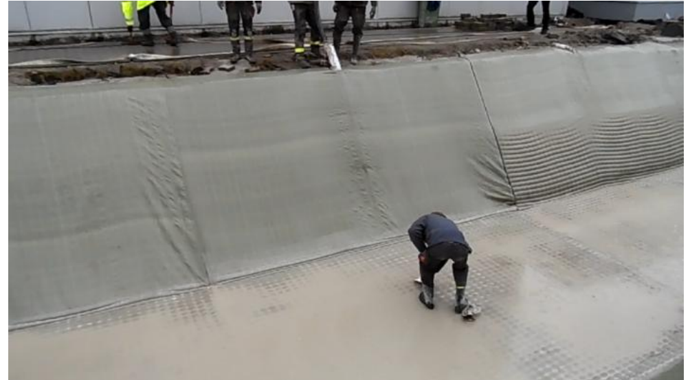
Incomat Standard filling (storm water pond)
