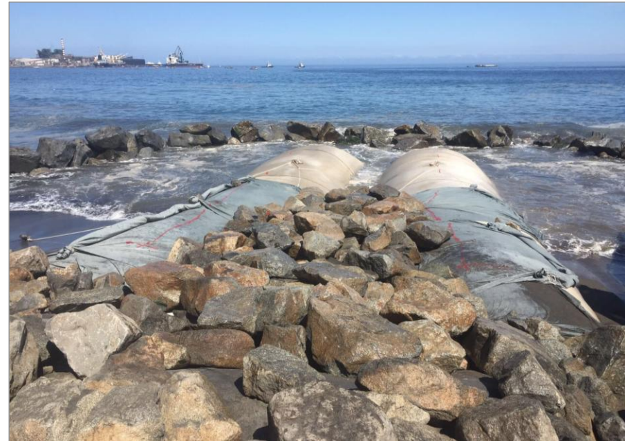
Installation of the rock cover (cushion layer of 0,3 to 0,5 tons; armour layer of 2 to 4, 4 to 6 and 6 to 8 tons rock)
