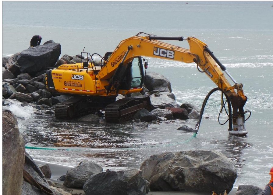
Use of a backhoe mounted slurry pump (type Dragflow, 140 m 3 /h) for tube filling
